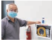
Installed AED device
