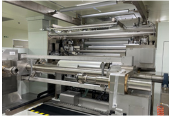
New coaters installed at the Agatsuma Plant
