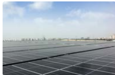
Solar power generation system
