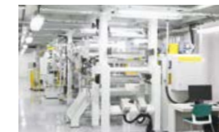
Large-scale pilot coaters in the Advanced Technology Building
