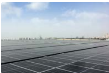
Solar power generation system
